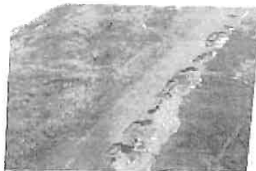
Before ARMORMAX - Levee Overlapping Failure
